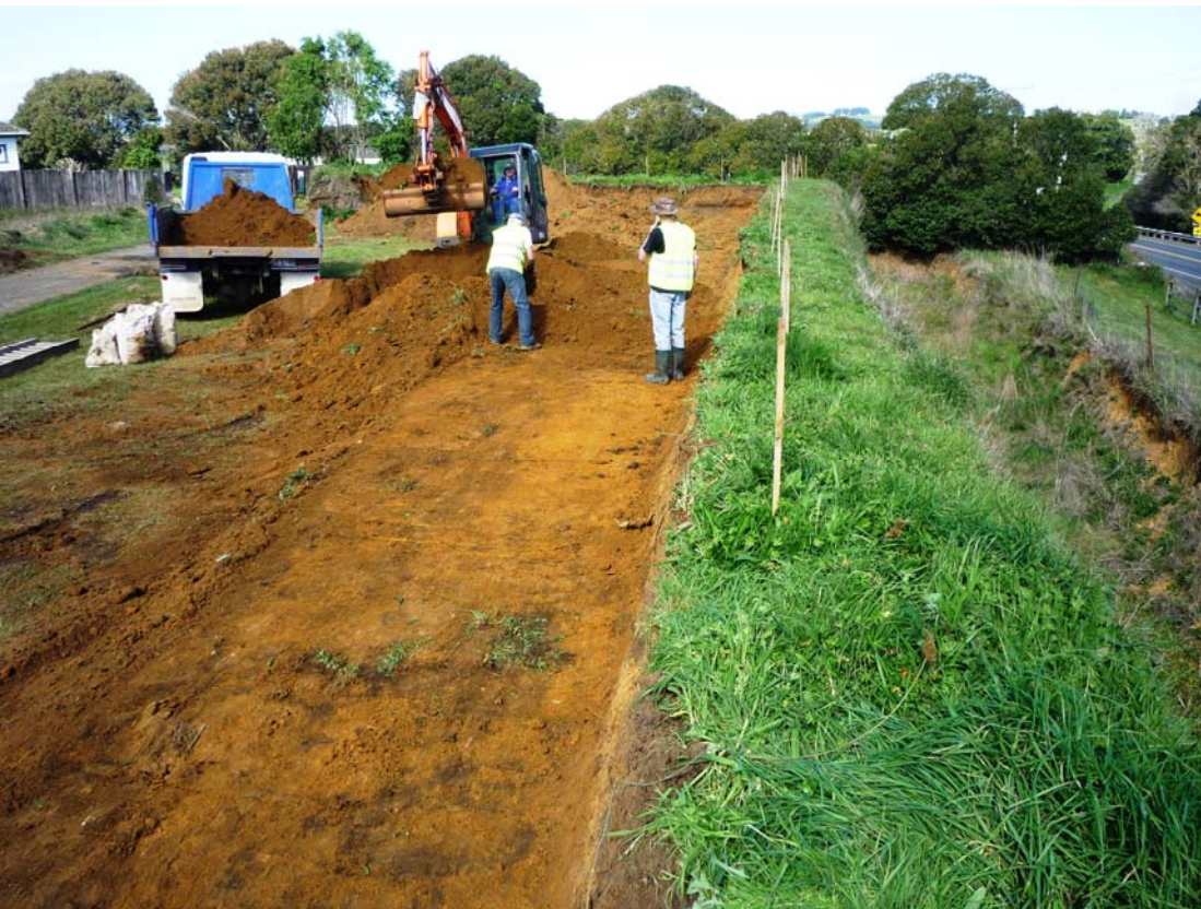
Cutting the firestep into west wall. The building is to be erected where the truck is parked.
